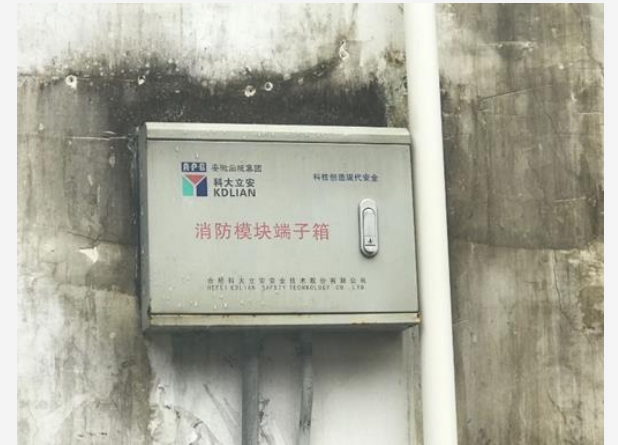
Fire-fighting module box
